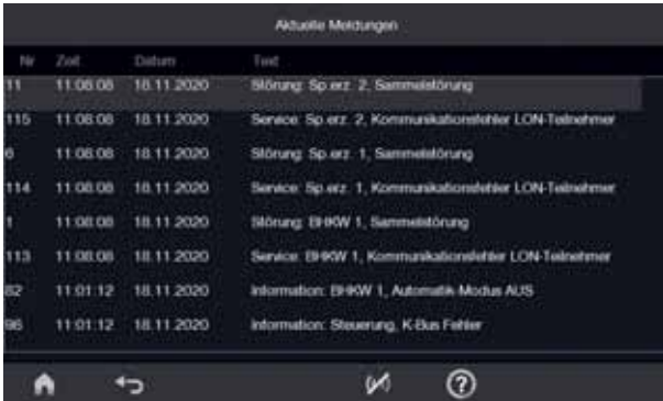
Messages from the connected heat generators and external pumps are displayed in plain text and as a list with the associated fault codes.
