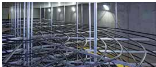
Interior view of an ice energy store.
