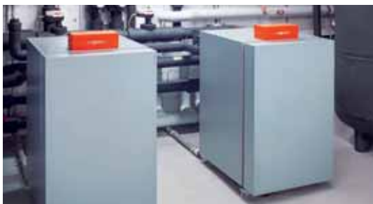
The Vitocal 300-G brine/water heat pumps each have an output of 12.6 kW.
