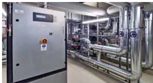
The Vitobloc 200 CHP unit supplies the electricity to operate the heat pump.
