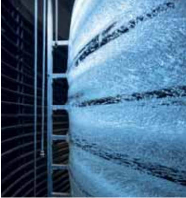
Water, as the storage medium, is harmless to the environment and can be used anywhere.
