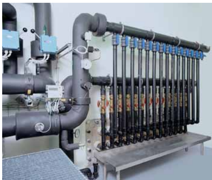
Geothermal probe manifold
