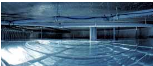
Interior view of an ice energy store – shown here in its frozen state.
